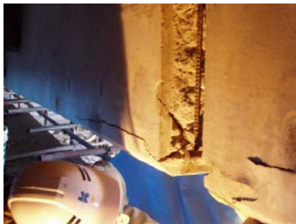
Photo 2: Corrosion induced cracking
