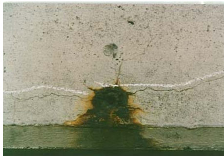
Photo 1: Damage to the main girder
