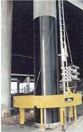
Figure 2: Automated FRP wrapping of a reinforced concrete bridge column (courtesy of Xxsys Technologies)
